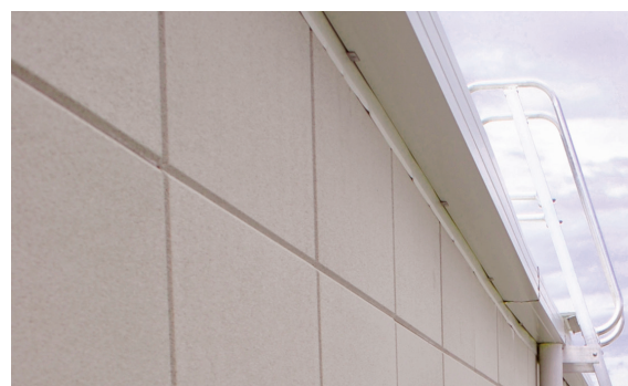
Regularly inspect flashing for functionality
