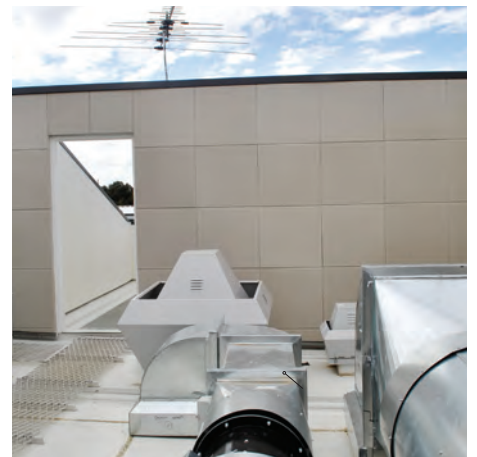
Cooling towers and HVAC
